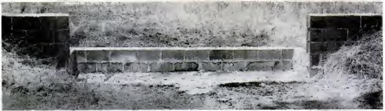
Concrete block toe wall, which is helping an Illinois farmer control erosion, was first modeled in toy blocks
